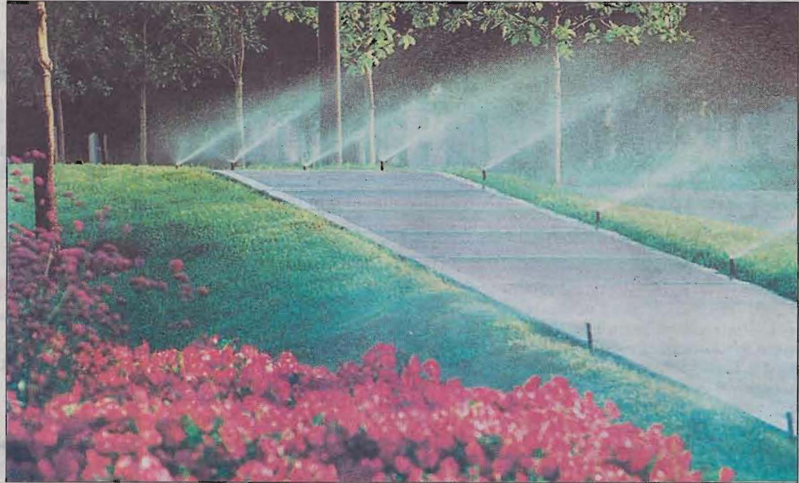
Irrigation system pop-up nozzles direct water onto a lush landscape.
